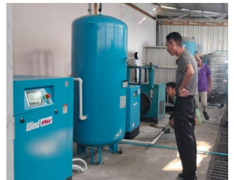
Compressed air system
